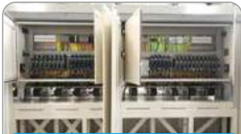
Isolated Electrical Cabinet
